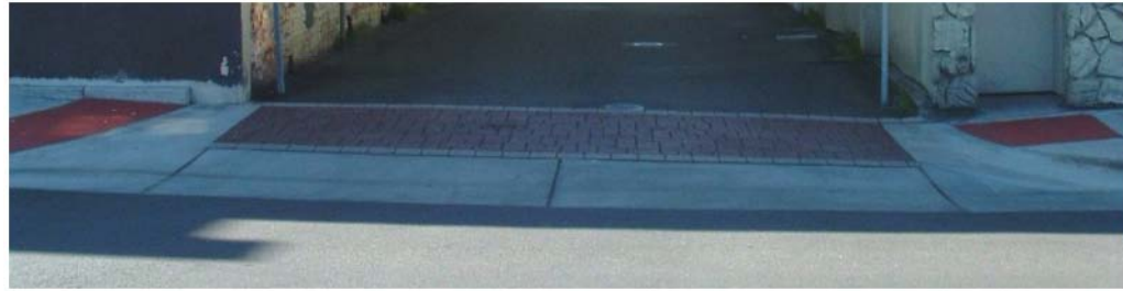
EXAMPLE IMPROVEMENT, N200D NORTH INTERSECTION LOOKING SOUTH ACROSS REDWOOD AVENUE, NEAR "MY BEAUTIFUL NAILS"
