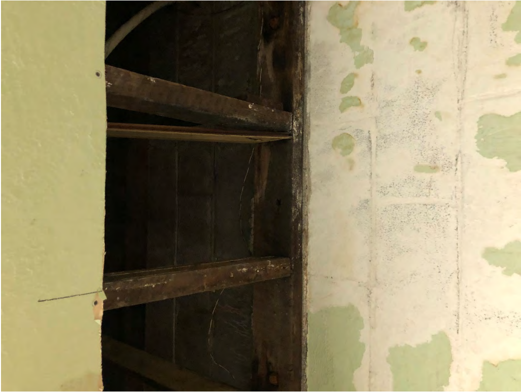
Fort Bragg Fire Station: Visual Deterioration/Damage from leaky roof
