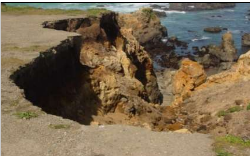
Photograph 3–18. Erosion and bluff undercutting at North Parkland bluff due to uncontrolled stormwater flows.
