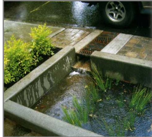
Stormwater planters allow roadway runoff to flow into and out of adjacent landscaping, where the stormwater is detained and treated.
